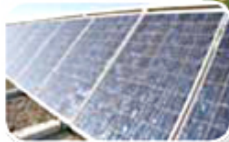
Solar panels on NOW roof
